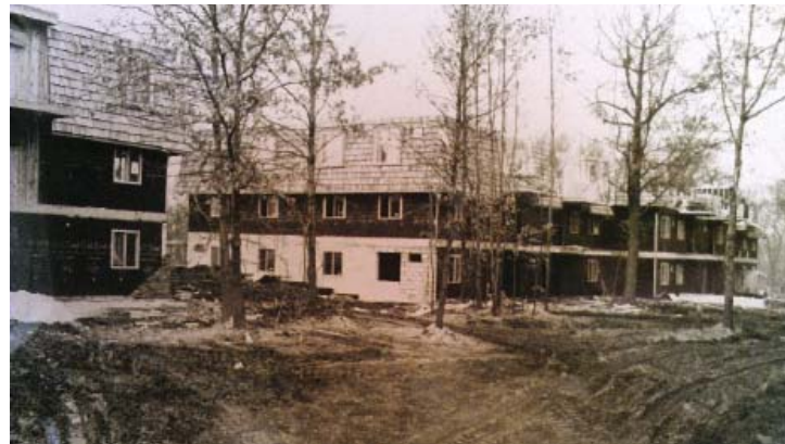
The final stages of the first buildings at the South Side of The Mansards.
